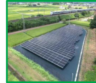
Power self-consignment system (Takashima City, Shiga Prefecture)
